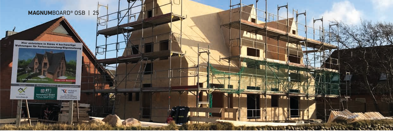
MMD, D-36163 Poppenhausen | Photograph: www.rosengruen.de
